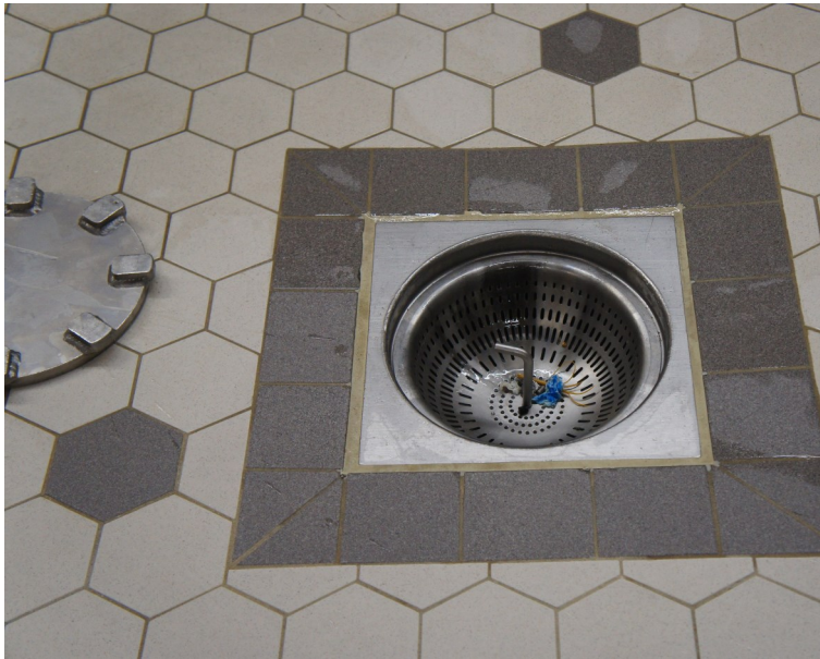
Above: Floor drain in brew house with mesh basket to capture waste grain
