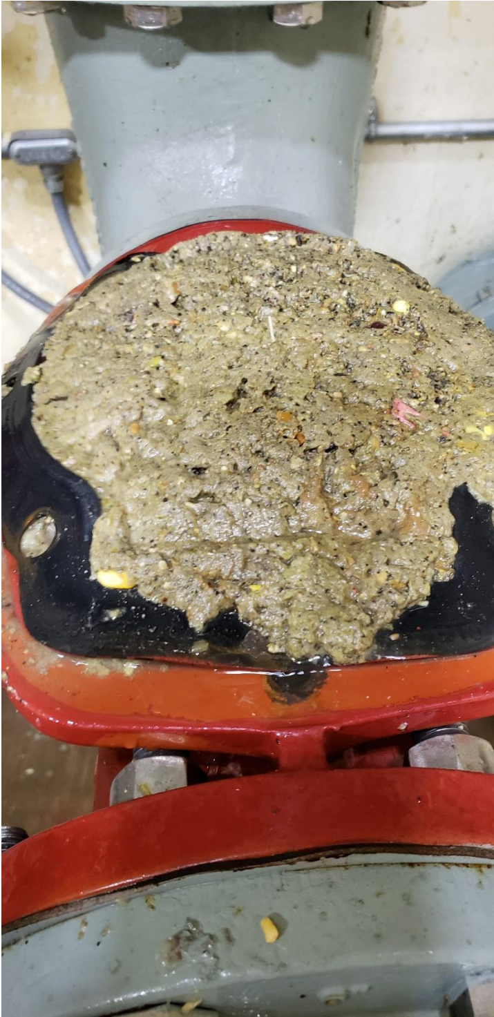
Blocked Check Valve from Brewery Operations Solids
