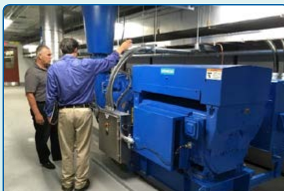
Paul Rodriguez (R), Senior Project Engineer at PWD, gives Efficiency Maine's Chuck Porter (L) a tour of the final installation.
